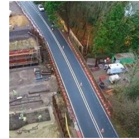
The £5.5 million replacement of a 114-year-old rail bridge on the A35 at Holmsley, New Forest.
